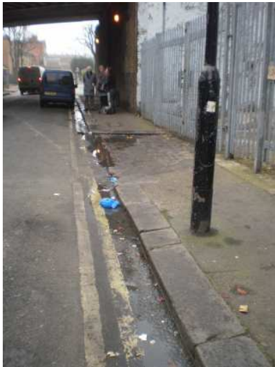
Pavement on the north side of the street east of the railway bridge.
